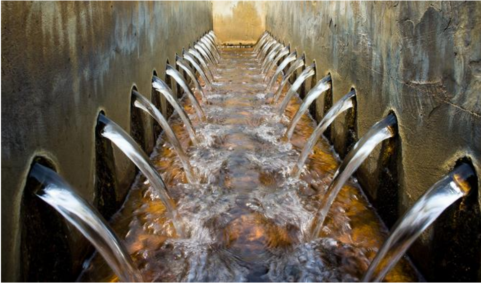
first independent sewage treatment plant (ISTP) (Arab News)
